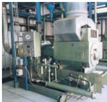
Four 1250 HP (930 KW) Turbo Air® Compressors installed at a glass facility.
