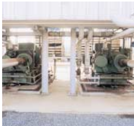
Two 1250 HP (930 KW) Turbo Air® Compressors installed at a chemicals facility.
