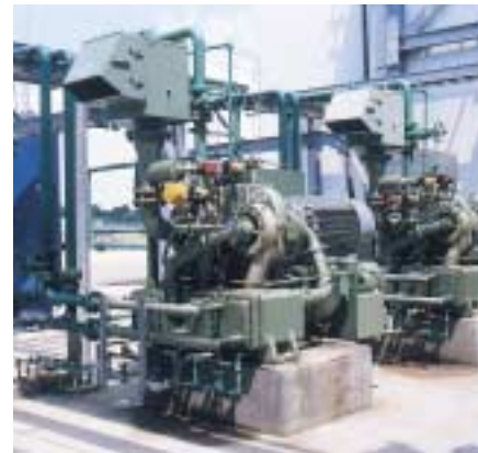
Two 200 HP (150 KW) Turbo Air® Compressors installed at a chemicals facility.
