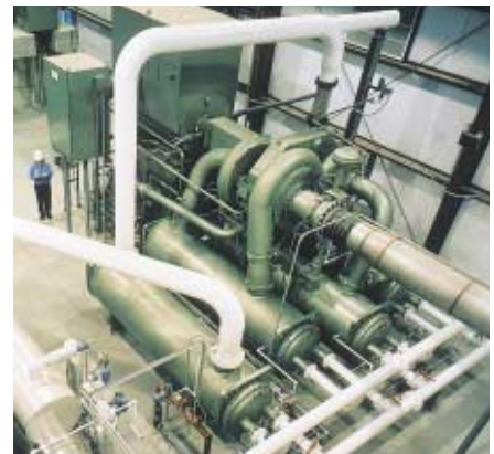
One 10,000 HP (7455 KW) MSG® Air Compressor installed at an air separation facility. One 11,000 HP (8200 KW) MSG® combination Nitrogen Feed/Recycle Compressor is also installed.
