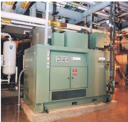
One 300 HP (225 KW) Turbo Air® Compressor installed at a major university for instrument air.
