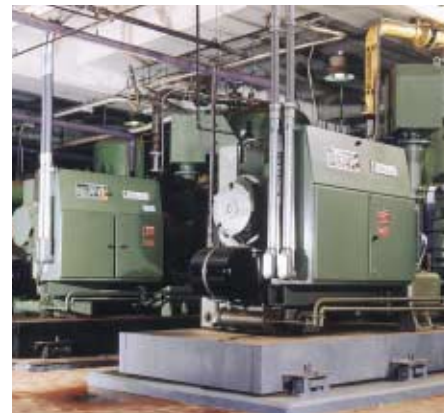
Two 300 HP (225 KW) Turbo Air® Compressors installed at a water treatment facility.
