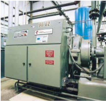
One 350 HP (260 KW) Turbo Air® Compressor installed at an automotive facility.
