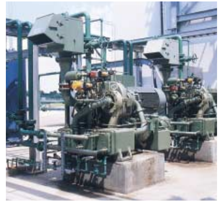
Two 200 HP (150 KW) Turbo Air® Compressors installed at a chemicals facility.
