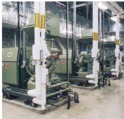
Three 200 HP (150 KW) Turbo Air® Compressors installed at an electronics facility. Three 500 HP (370 KW) Turbo Air® Compressors are also installed.
